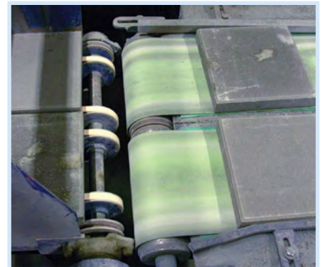
FK - 3 Brick pre - oven conveying
